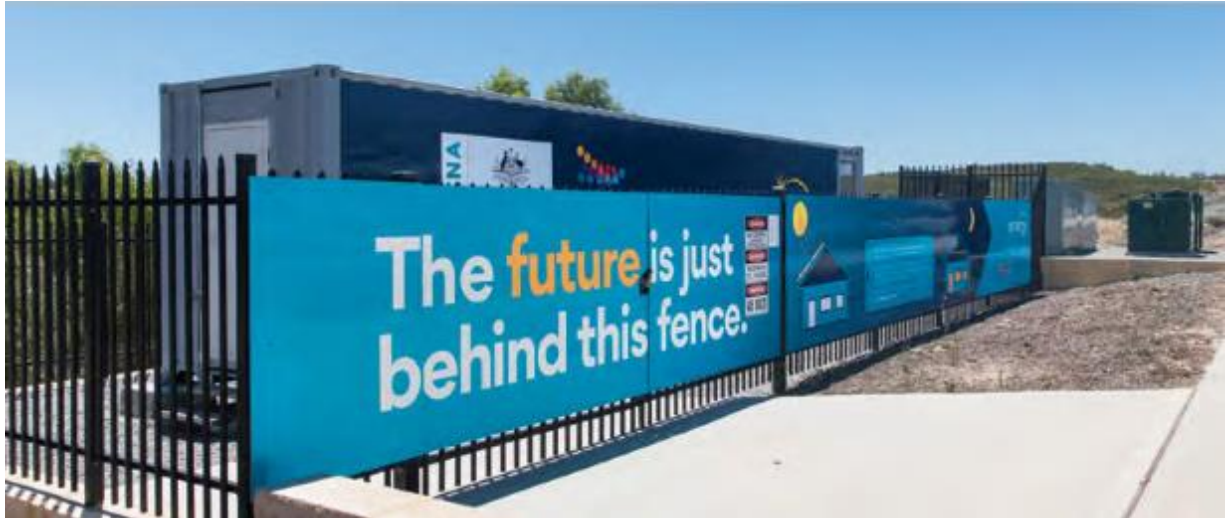
Figure 11: Alkimos Beach 1.1 MW battery in WA
